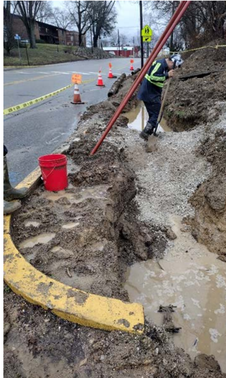
Rural utility works battling leaky infrastructure.
