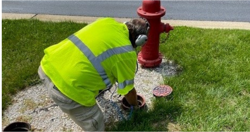
Chad Reynolds conducting a leak audit in the Town of Middlebury, IN.
